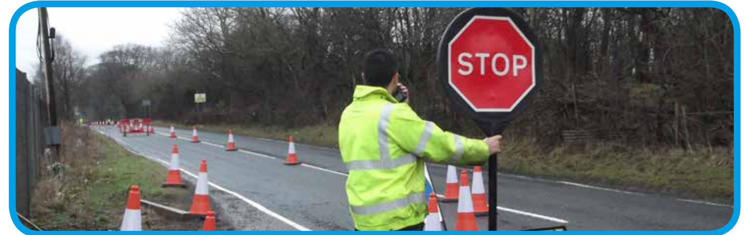
Defect and Priority Table 7:
